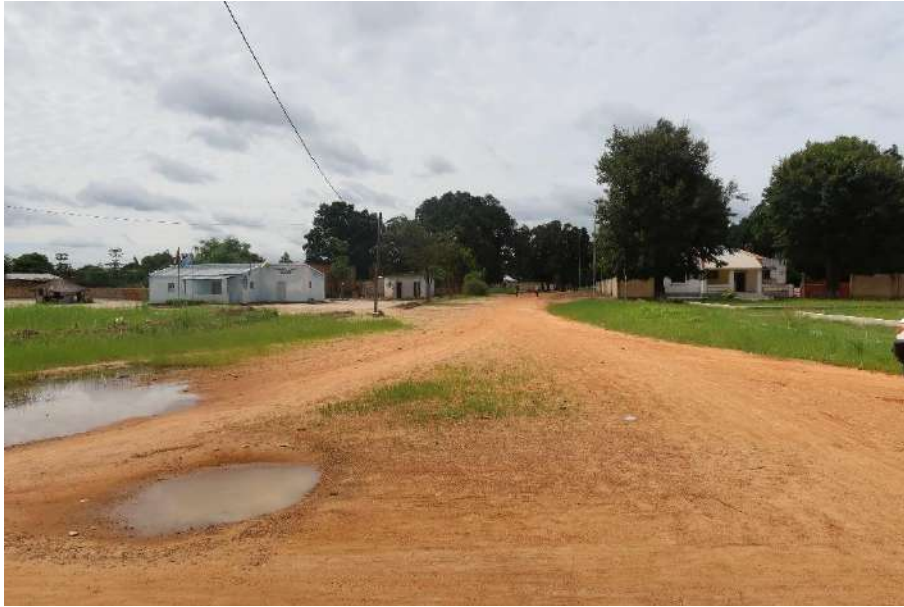
Figure 8 – Photographic record of the beginning of the road section between Cazombo and Lumbala Caquengue located at PK 0+000.
