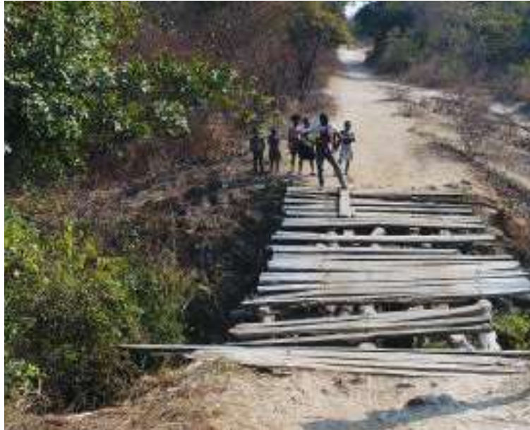
Figure 16 – Photographic record of the bridge located at PK 52+700 (Source: QG Konstruktion GmbH).
