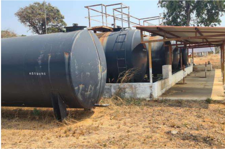
Figure 39 – Fuel tanks at the project support site (Source: QG Konstruktion GmbH).
