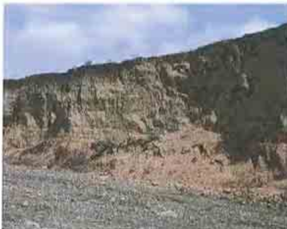
Photo 3: Over 10m high fragile left bank of Ajewa R. just at upstream of RW crossing point
