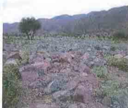
Photo 4: An example of heavy siltation and boulders accumulation at -stat. 45+500 crossed by the RW line
